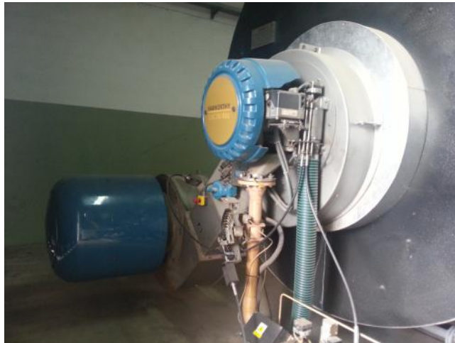
Fig. 2. Propane gas burner in a steam boiler.
