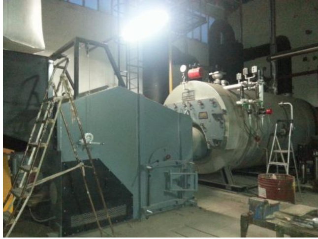
Fig. 4. Biomass burner in a steam boiler using wood pellets.
