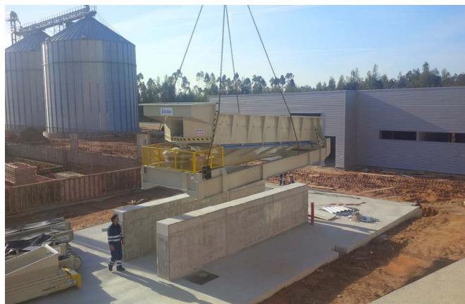
Figure 3. Biomass torrefaction plant with an annual capacity of 100,000 t/y being built in Portugal.
