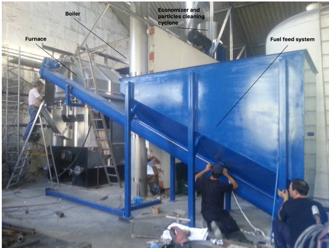
Figure 1. Fitting of a steam boiler that uses wood pellets as fuel. The boiler production capacity is equal to 2t/h steam at 10 bar.
