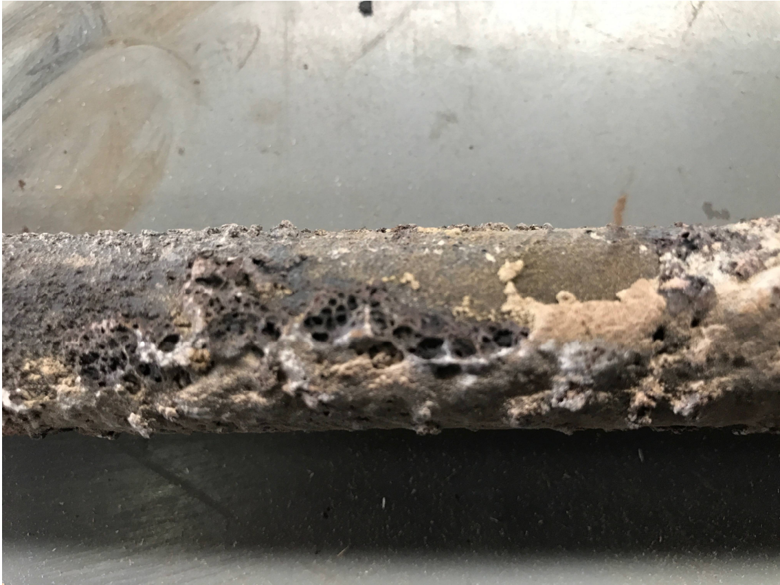
Figure 2 - Slagging and fouling phenomena in the surface of a temperature probe of a biomass boiler.
