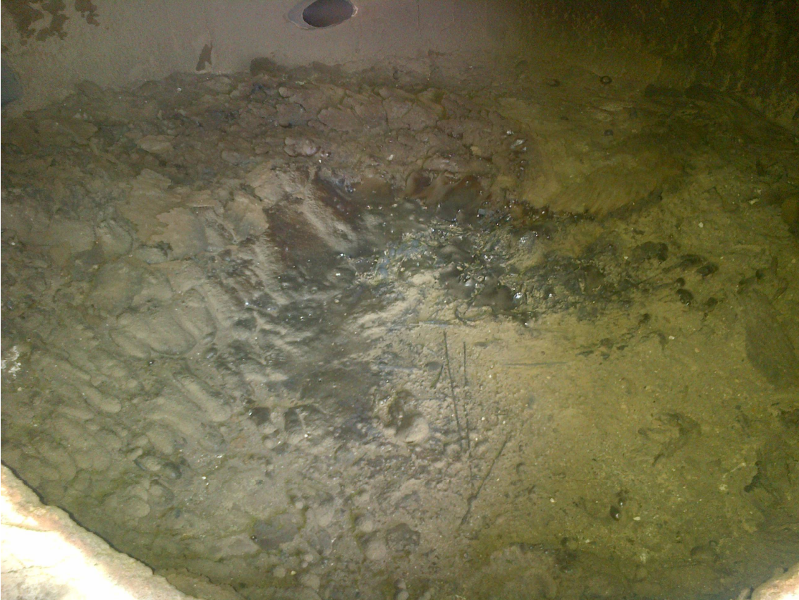
Figure 1 – Melted ashes deposit in a biomass boiler furnace that uses pulverized sawdust as fuel.
