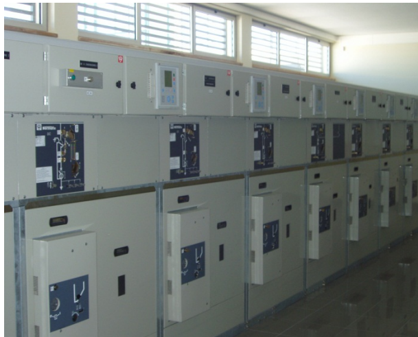
Fig. 11. Inside the control house of the wind farm.
