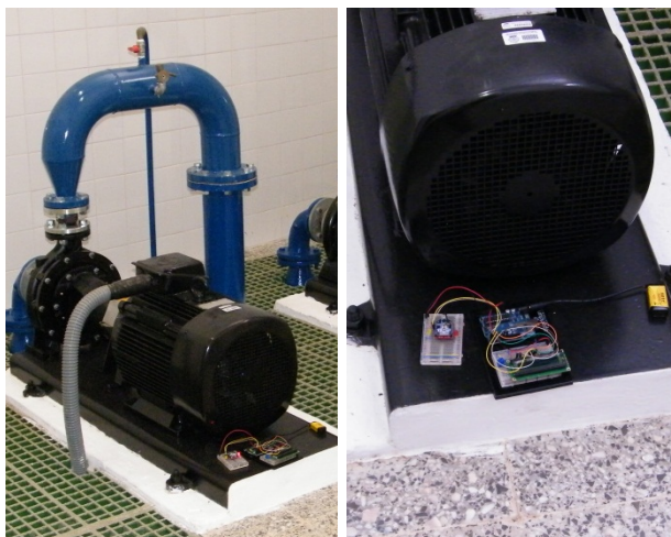
Fig. 8. Inside the water supply installation (on the left) with the ZigBee coordinator suitably placed (on the right).
