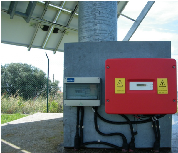
Fig. 7. Inverter used for the grid connection.
