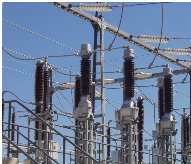
Fig. 12. Outdoor substation environment.
