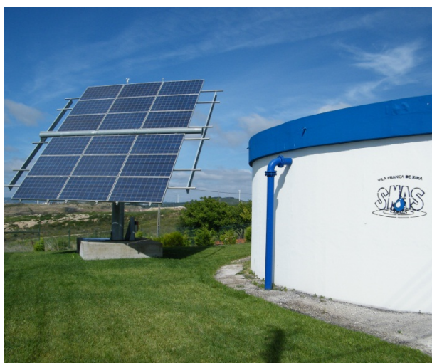
Fig. 6. Photovoltaic energy system belonging to the water treatment and distribution system (SMAS) operator.
